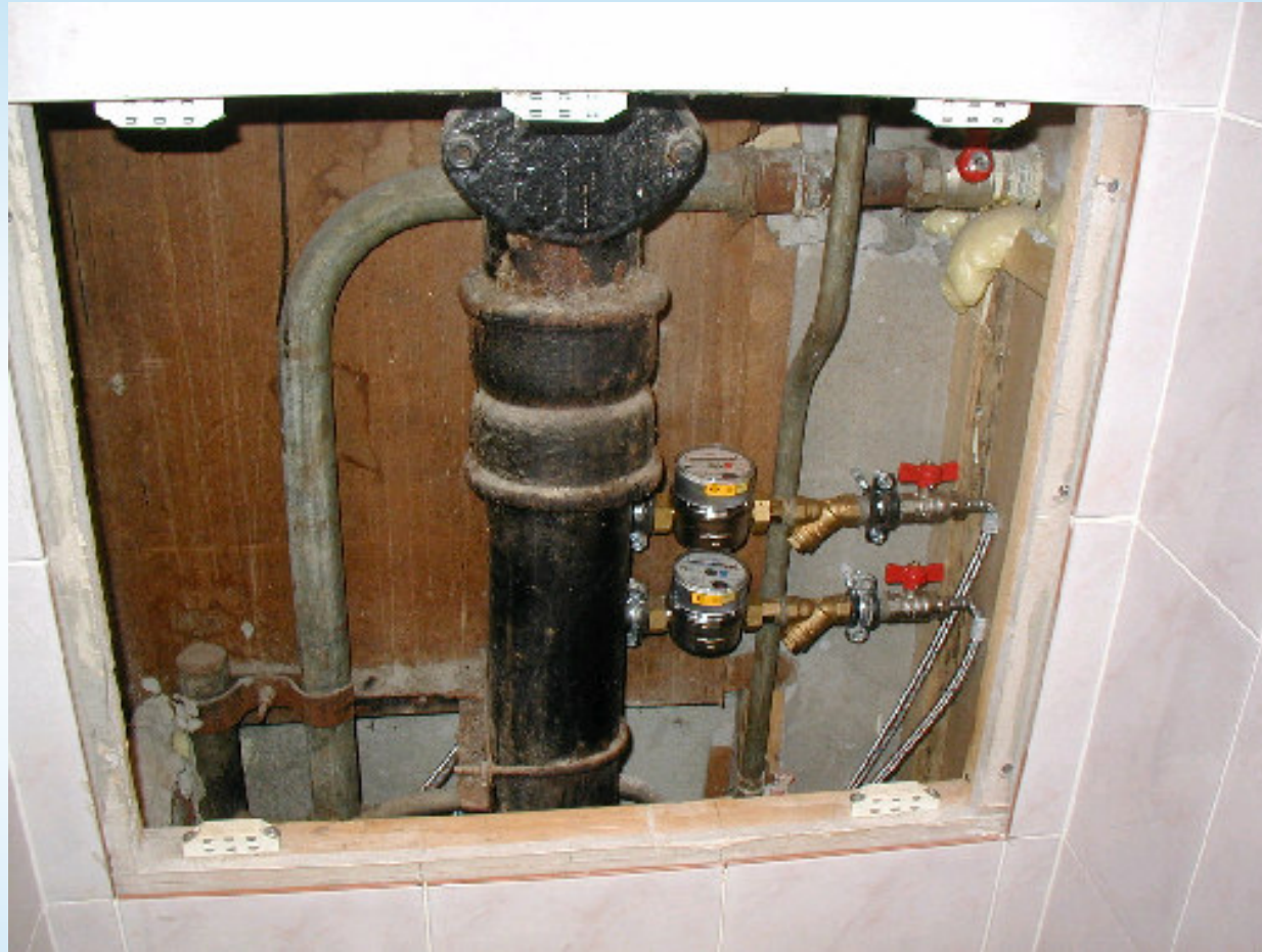
Fig. 30: Individual hot and cold water meters installed in a flat
