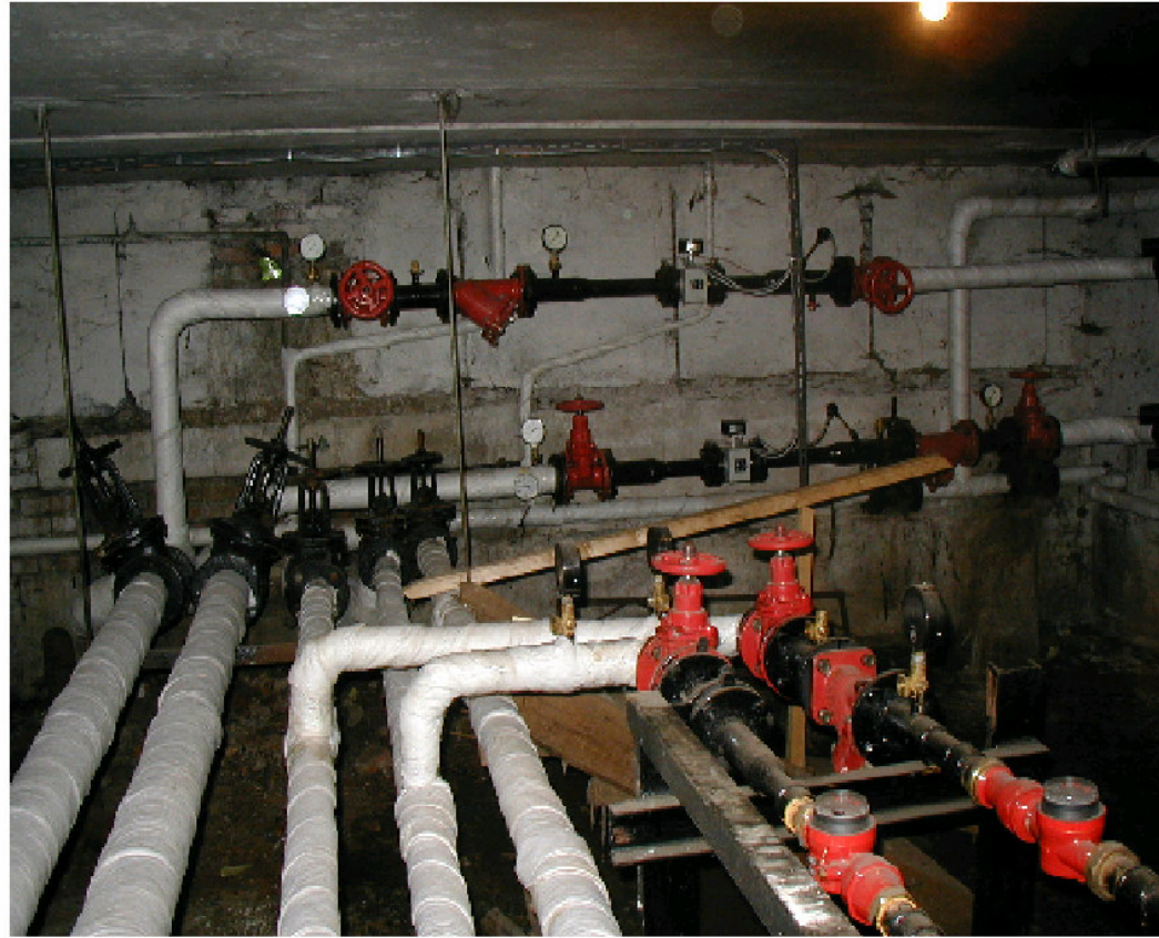
Fig. 28: Pipe insulation, valves, building level heat and water meters installed at a building
